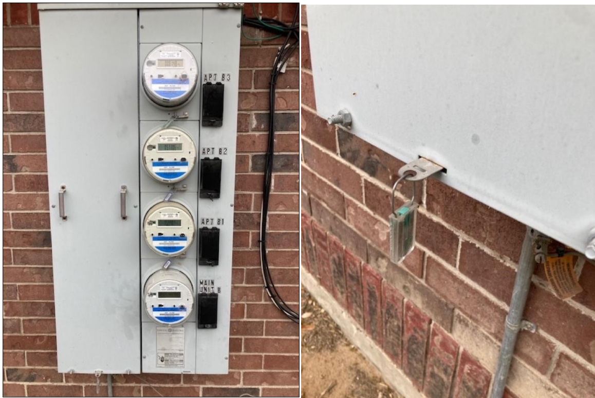
Figure 4. Building B meter bank—note additional meter for common area loads. Left side of panel is locked by the utility.
